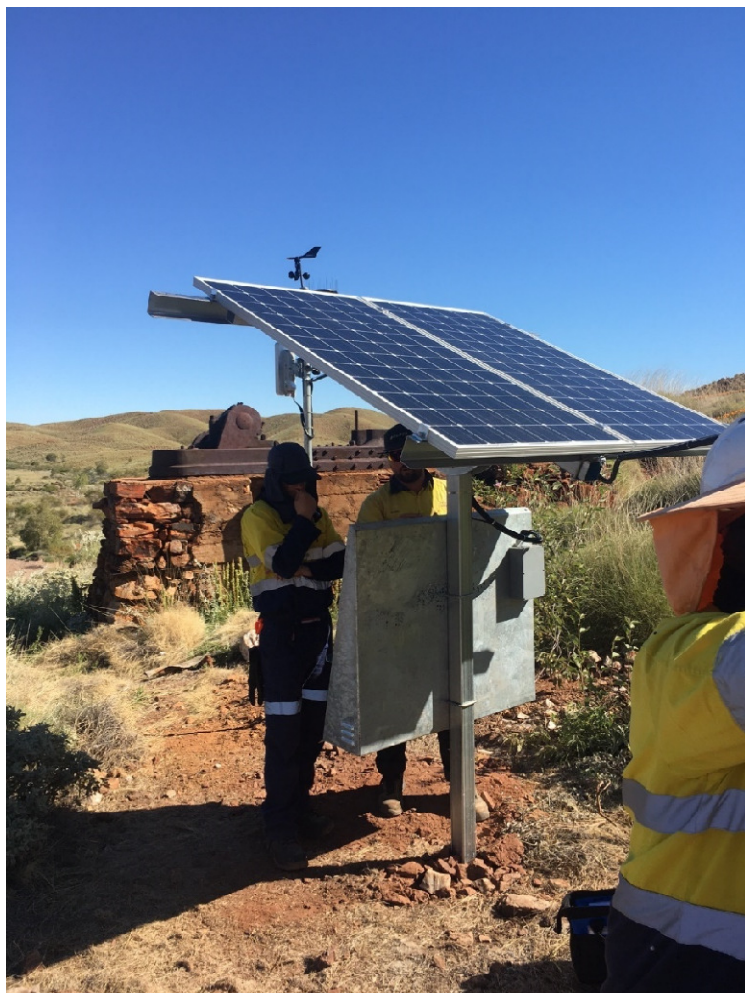
Permanent blast monitoring station at Klondyke Queen
